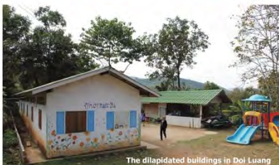
The dilapidated buildings in Doi Luang
