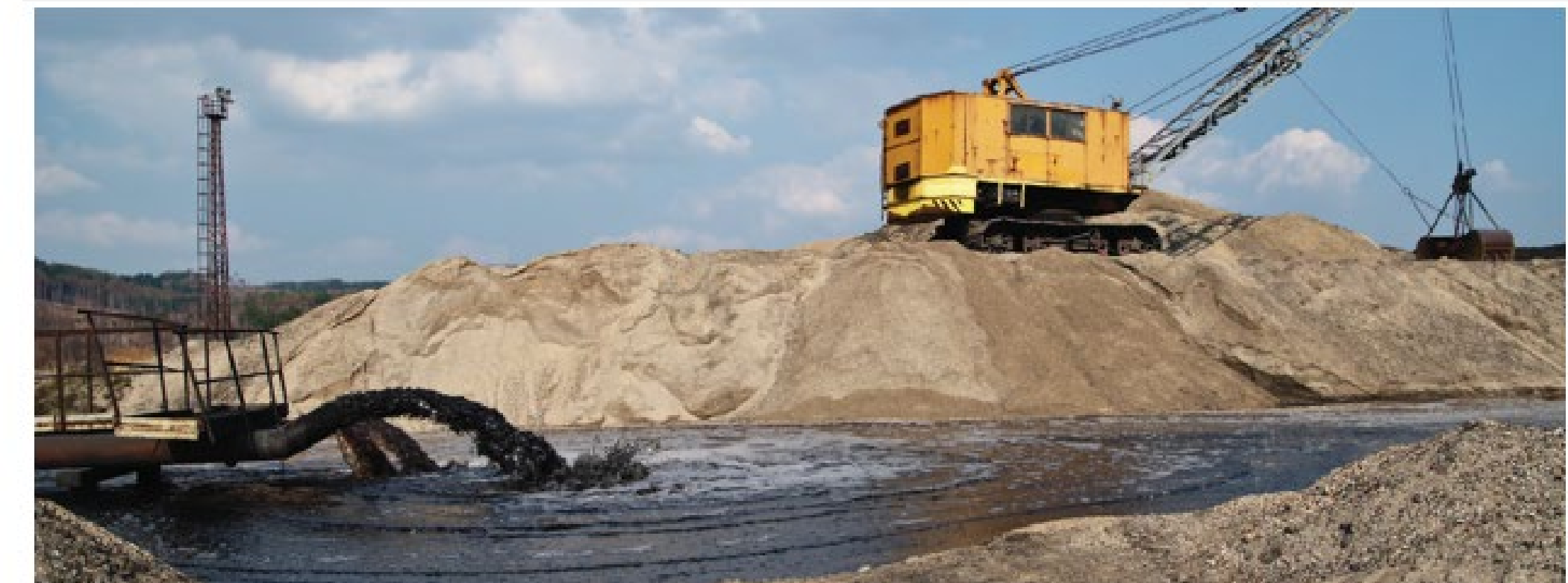
Heavily Contaminated Sludge Treatment
