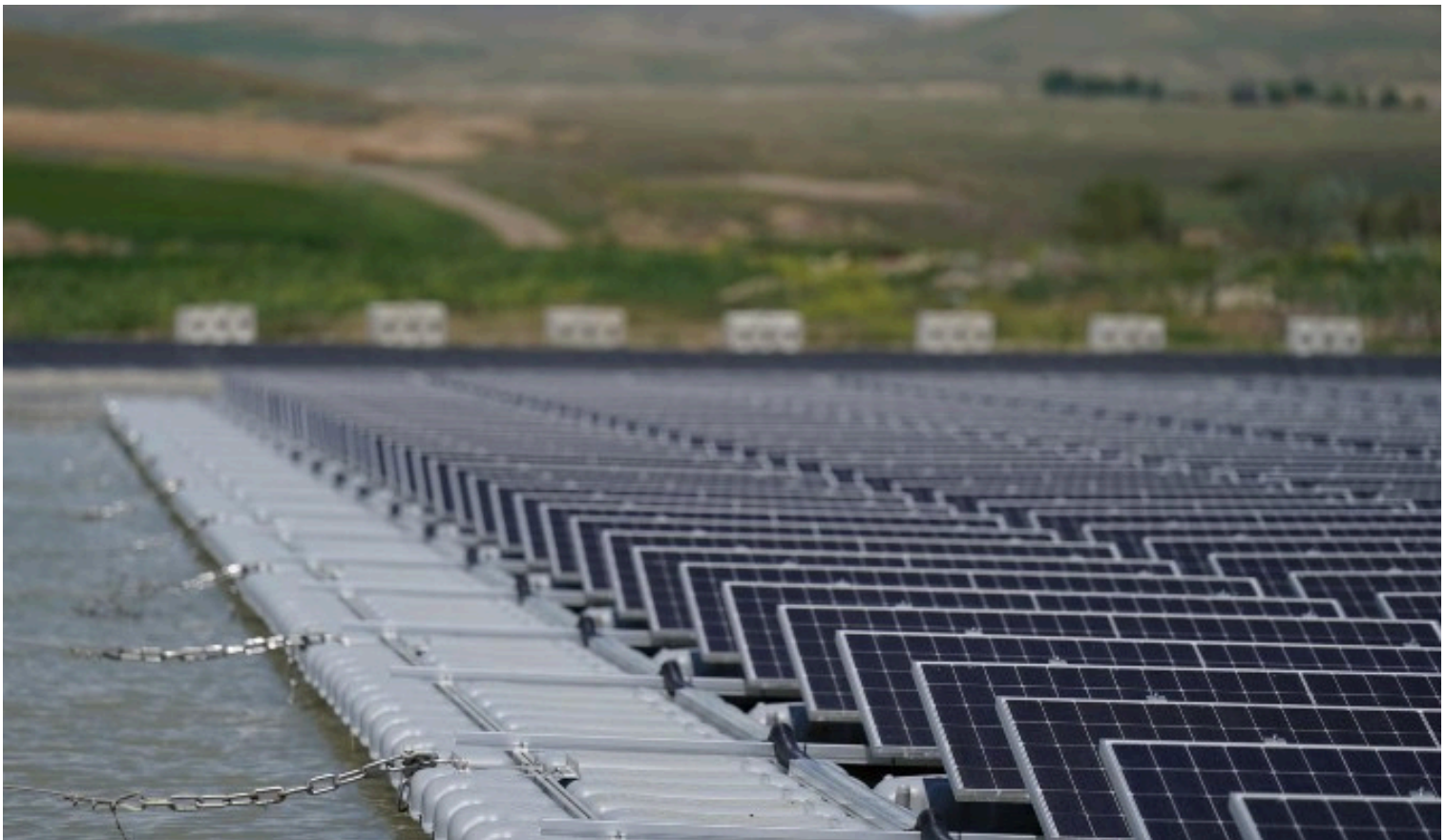
Garbadani floating photovoltaic power plant. Agenda.ge
